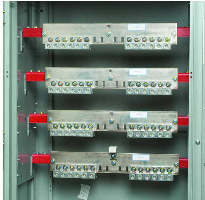
Mechanical Lug Terminations Shown
