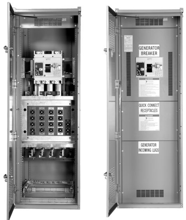
Typical Generator Quick Connect Switchboard (Typical of 1600 A) Shown with Covers Removed (Left) and In-place (Right)
